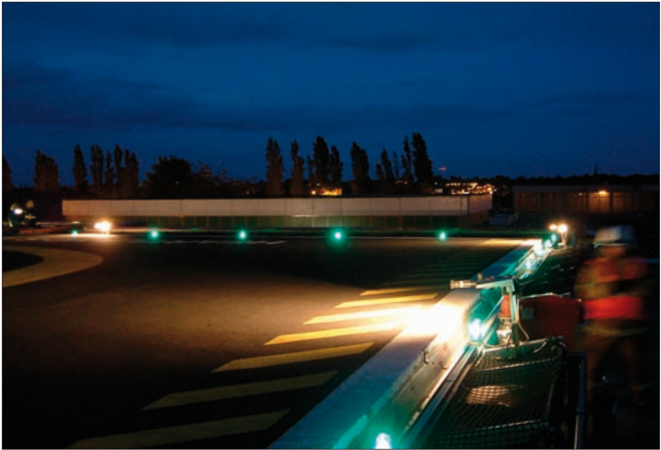
Green perimeter and xenon floodlights on an elevated helipad at Birmingham Heartlands Hospital
